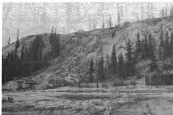
Figure 15. Extensive sloughing on slope has completely obliterated access road at its upper end, May 1957 (DBR photo BR 6771)
